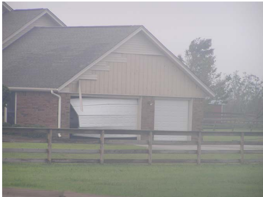
Garage door and siding damage to a home near Winnie, TX. Photograph taken 2:00 pm CDT September 14, 2008. Photograph by Tanya Brown.
