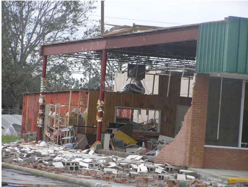
Damage to a structure adjacent to the Dairy Queen in the previous photo. Note the unattached brick/cinderblock façade. Photograph taken on the afternoon of September 15, 2008 by Tanya Brown.
