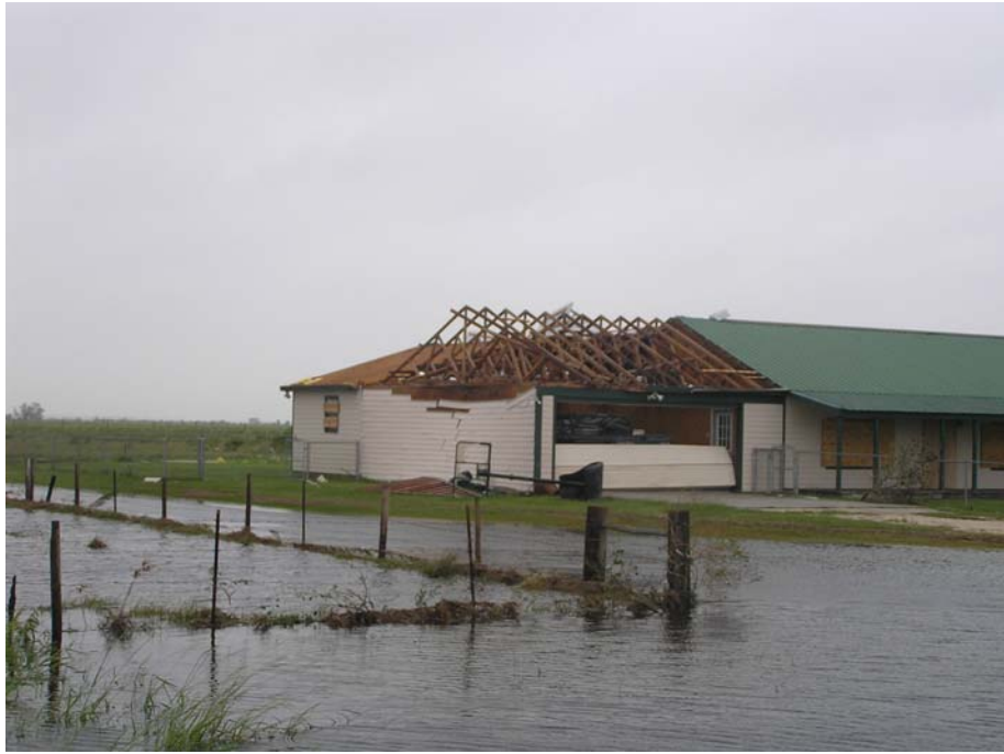
Roof decking loss and garage door failure near Winnie, TX. Photograph taken 3:00 pm September 14, 2008. Photograph by Tanya Brown.
