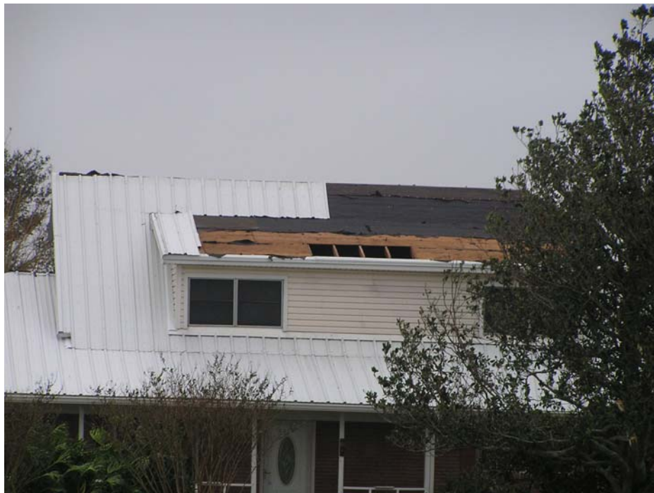
Roof decking loss and metal roof loss in Winnie, TX. Photo was taken looking north at the south facing front of the residence. Photo was taken during the afternoon of September 14, 2008. Photograph by Tanya Brown.
